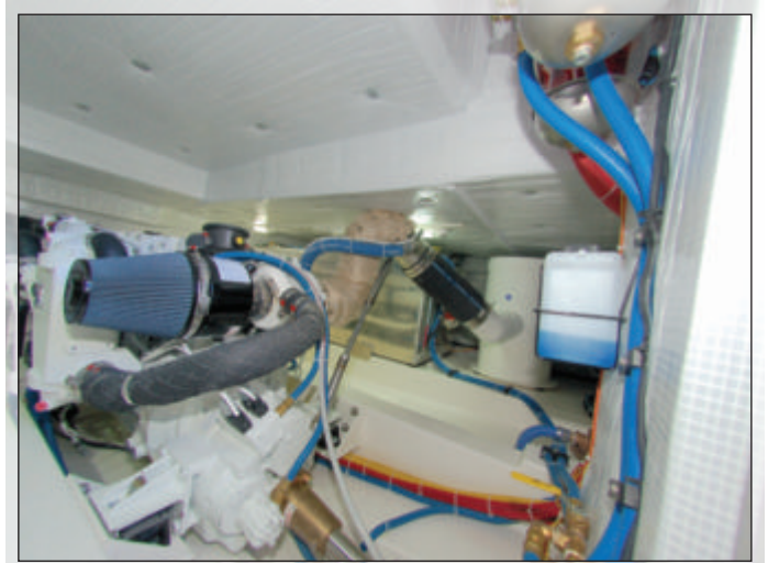
The engine room features excellent access, room to work, and thick sound insulation.
